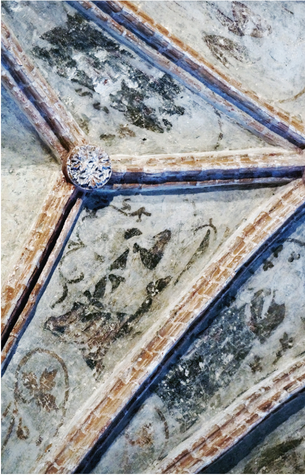
Fig. 9. Part of the northern bay vault with traces of exposed polychrome (2 nd quarter of the 15 th century?) (photo by A. Piwek)
