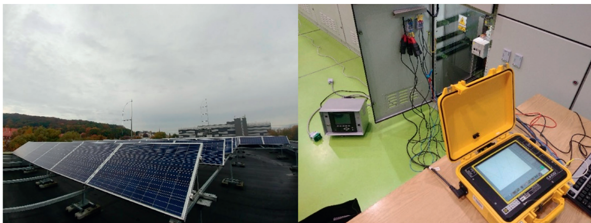
Photo 1. Pictures of a) tested photovoltaic plant (left) b) measuring station (right)
