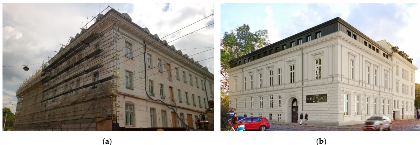
Figure 1. Former Leipziger Palace in Wrocław: (a) view on the facade during reconstruction; (b) facade visualization after reconstruction to the hotel building.
