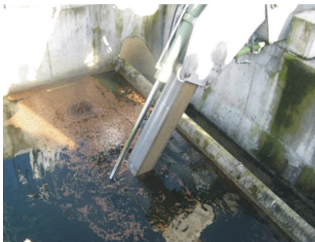
Figure 1. Purification of water from “thick” pollution at an SHP (photography: B. Igliński).
