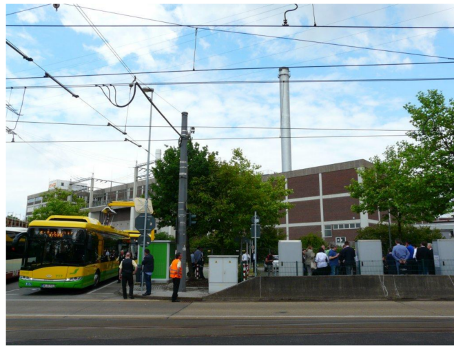
Figure 3. Charging station for electric bus and electric cars powered from the tram overhead line in Oberhausen, Germany.
