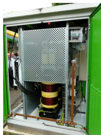
Figure 4. DC/DC converter used for powering a charging point for electric buses and cars from a tram overhead line in Oberhausen, Germany.
