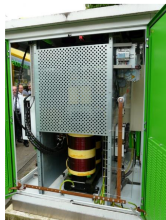
Figure 4. DC/DC converter used for powering a charging point for electric buses and cars from a tram overhead line in Oberhausen, Germany.
