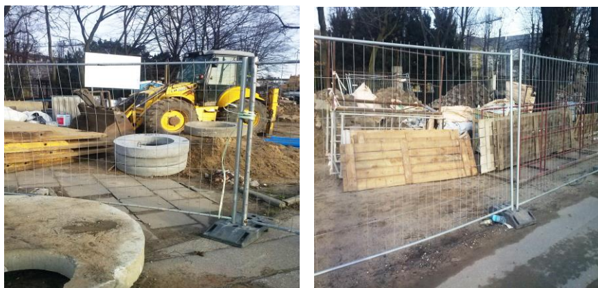
Fig. 1. Examples of elements of the building site and site compound protected in a reckless and inappropriate manner
