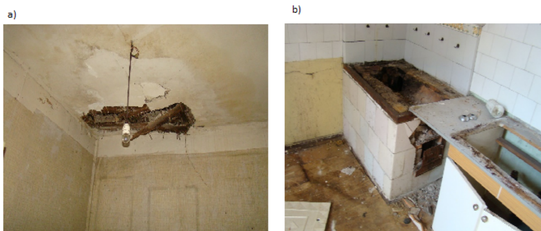
Figure 12. Building planned for modernization – lokale mieszkalne: a) broken ceiling above the ground floor, b) depreciation of equipment
