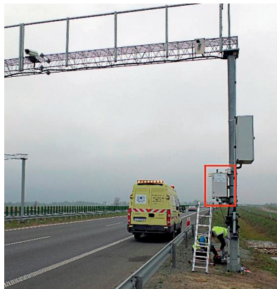
Fig. 30.1. Measuring station (marked with a red rectangle) mounted on the gantry pillar
