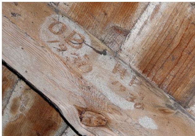
Figure 3. A rafter at the top of the roof of the monastery's west wing. (Hliwiadczyń, Cholewska, and Grunwald 2018).
