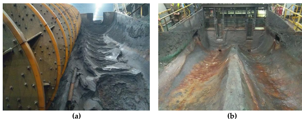
Figure 2. Preparation for anode installation: (a) view of the classifier with dismantled spiral; (b) view of the classifier with two dismantled spirals and feed removed from inside the tank.
