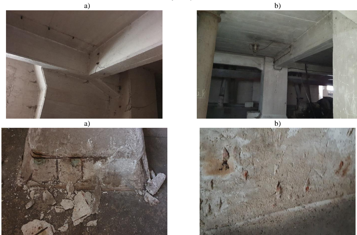
Photo 6: Grain Elevator building - level -1: a) mechanical damage to structural elements, floor zone: c) concrete cover falls off the column heads at the level of the foundation slab, d) moisture in the outer wall
