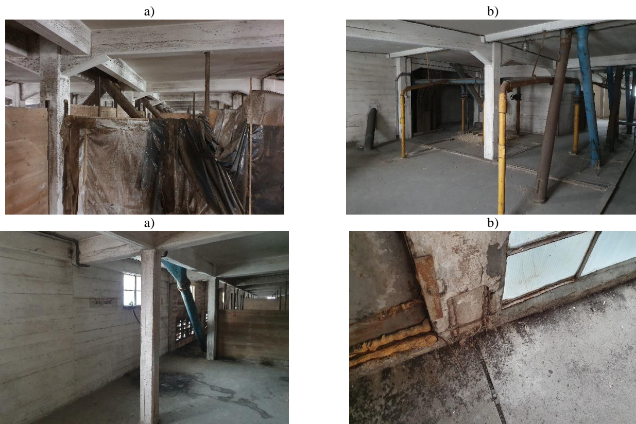
Photo 4: Grain Elevator building - level +7: a), b), c) division of the usable area with wooden partitions, d) falling off the concrete cover in the floor zone
