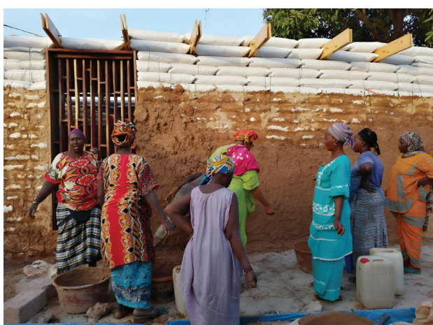
Fig. 2. Polyvalent Cultural Centre, Tanaff, Senegal. Processing of sack walls with earth mortar
