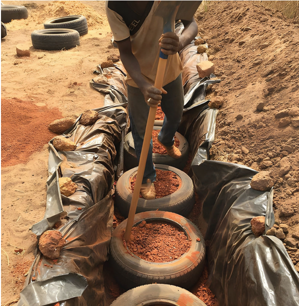
Fig. 5. Primary School, Quartier Dixième, Thiès, Senegal. Foundations made of tires filled with soil (source: image courtesy Let's build my school – humanitarian organization)
