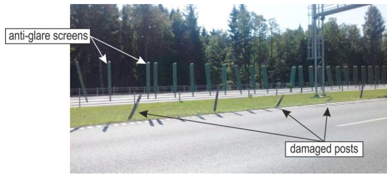
Fig. 2 Photograph of a damaged cable barrier with anti-glare screens (source: GDDKiA, Poland).
