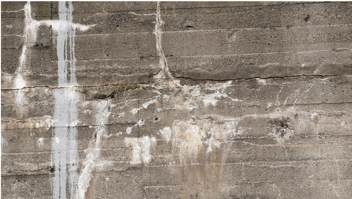
Photo 2: Examples of calcium carbonate leaks on the south-west elevation (external gable (transverse) wall from the land side (left)) of the Bunker building
