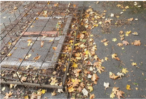
Photo. 8: No bumpers (bumpers) in front of the windows next to the windows on the roof above the former office spaces (A)
