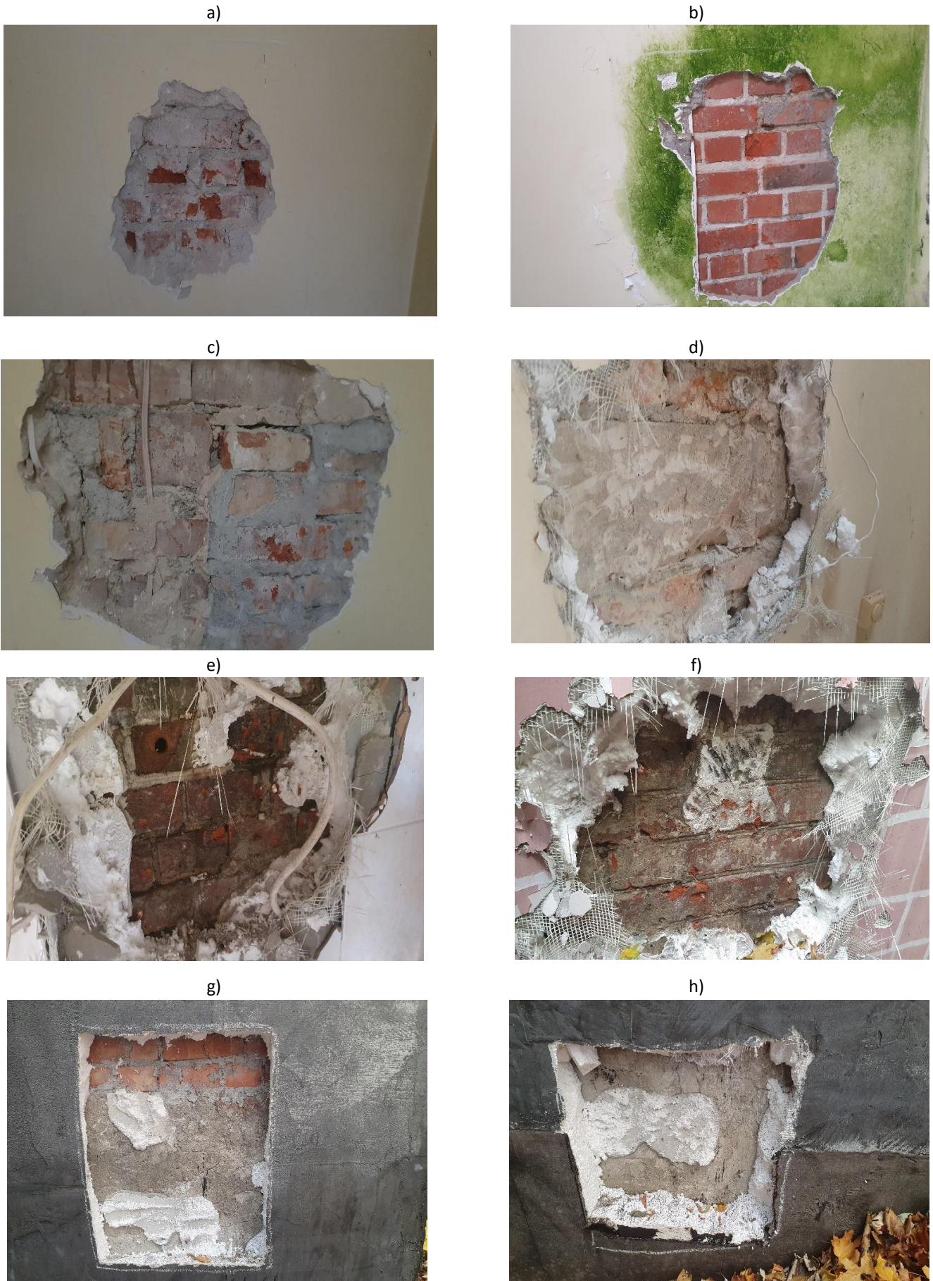
Photo. 9: View of the outer wall (from the escarpment side) of the former office rooms (A): a) O1, b) O2, c) O3, d) O4, e) O5, f) O6, g) O7, h) O8, i) O9, j) O10, k) O11
