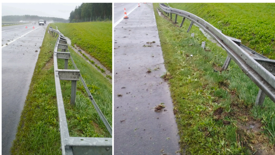
Fig. 12. General view of the accident no 2, source of photo: GDDKiA, Poland.
