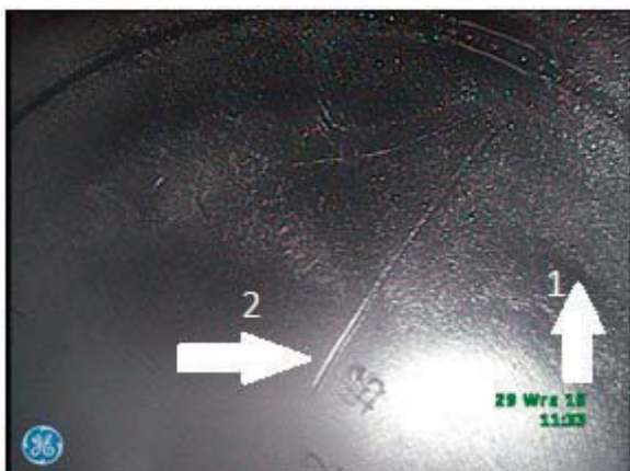
c) Piston crown – visible traces of carbon deposits (1) and scratches on the surface (2)
