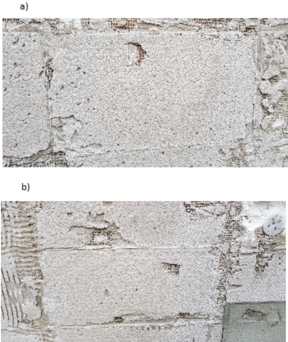
Figure 3. Mechanism a), b) (method of detaching) the ceramic cladding of the building facade
