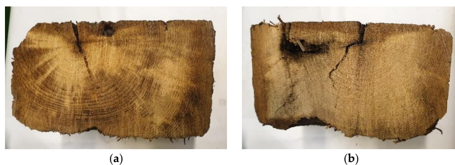
Figure 1. Cross section of the tested tie through the center of length (a) and 1 cm from the edge (b).
