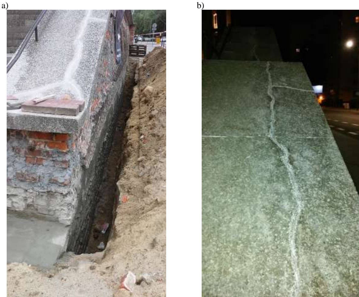
Photo 14. The wall at the entrance from the west elevation (along 3 Maja Street) during renovation works: a) dismantled cracked stone cladding and implementation of vertical damp-proof insulation, b) repaired cracks in the terrazzo cladding of the wall cap (names of the street as of 2023) (photo by Jacek Bramorski)
