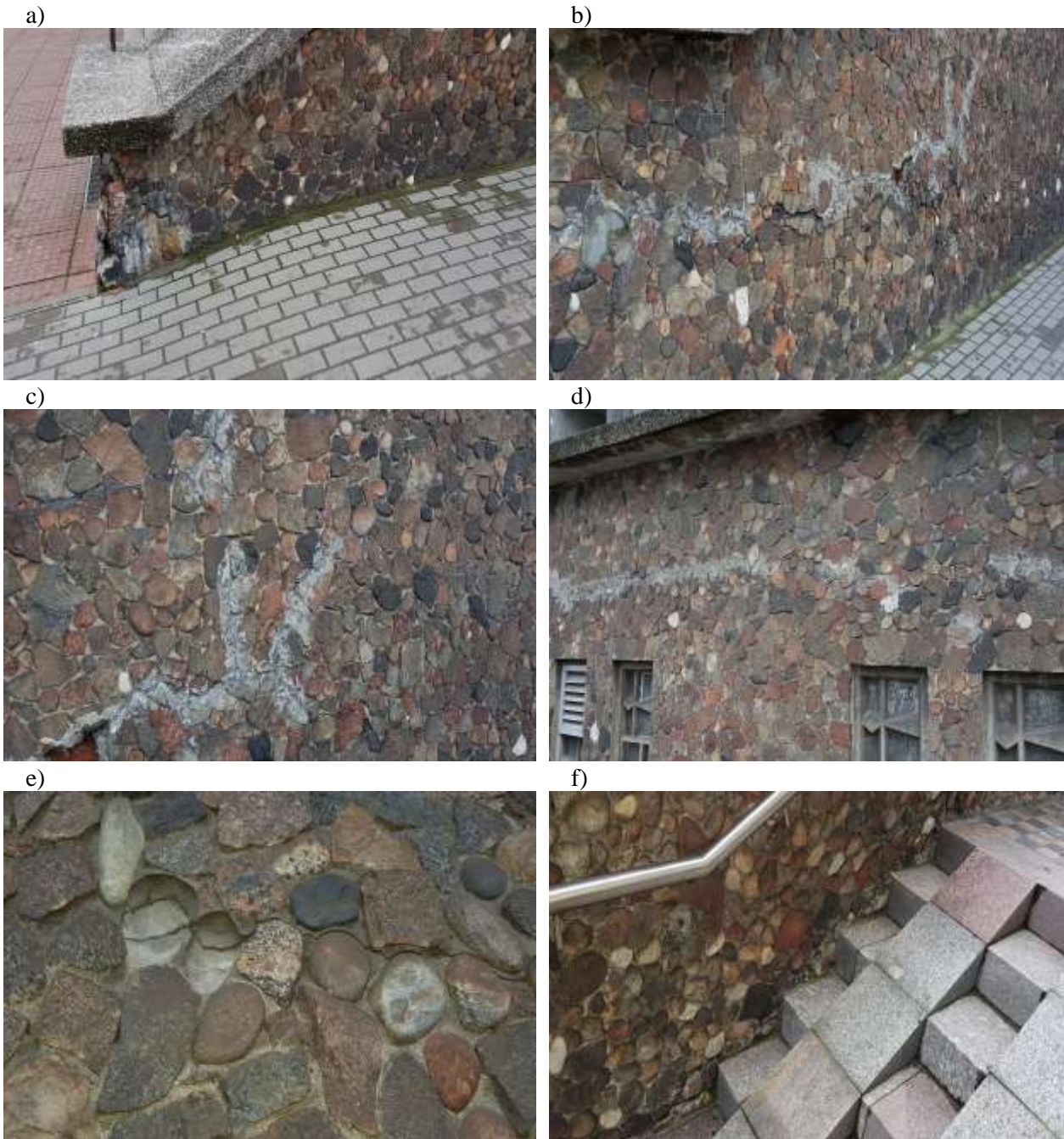
Photo 12. Damage to the stone cladding of the wall at the entrance from the west elevation (along 3 Maja Street): a), b), c), d) wall cracks, e) stone falling out from the outside, f) cracks from the inside (street names as of 2023) (photo by Maciej Niedostatkiewicz)
