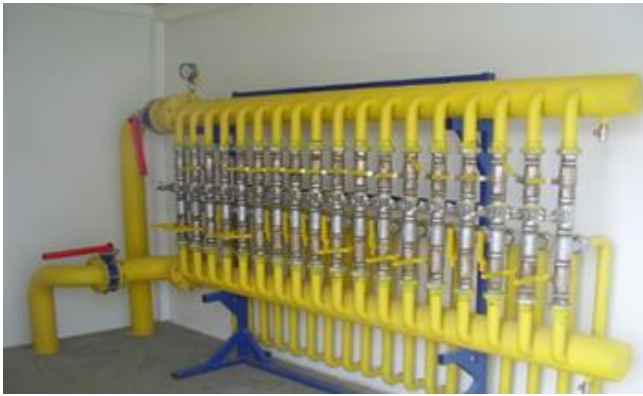
Fig. 3. Connection of gas wells to main pipelines (13)
