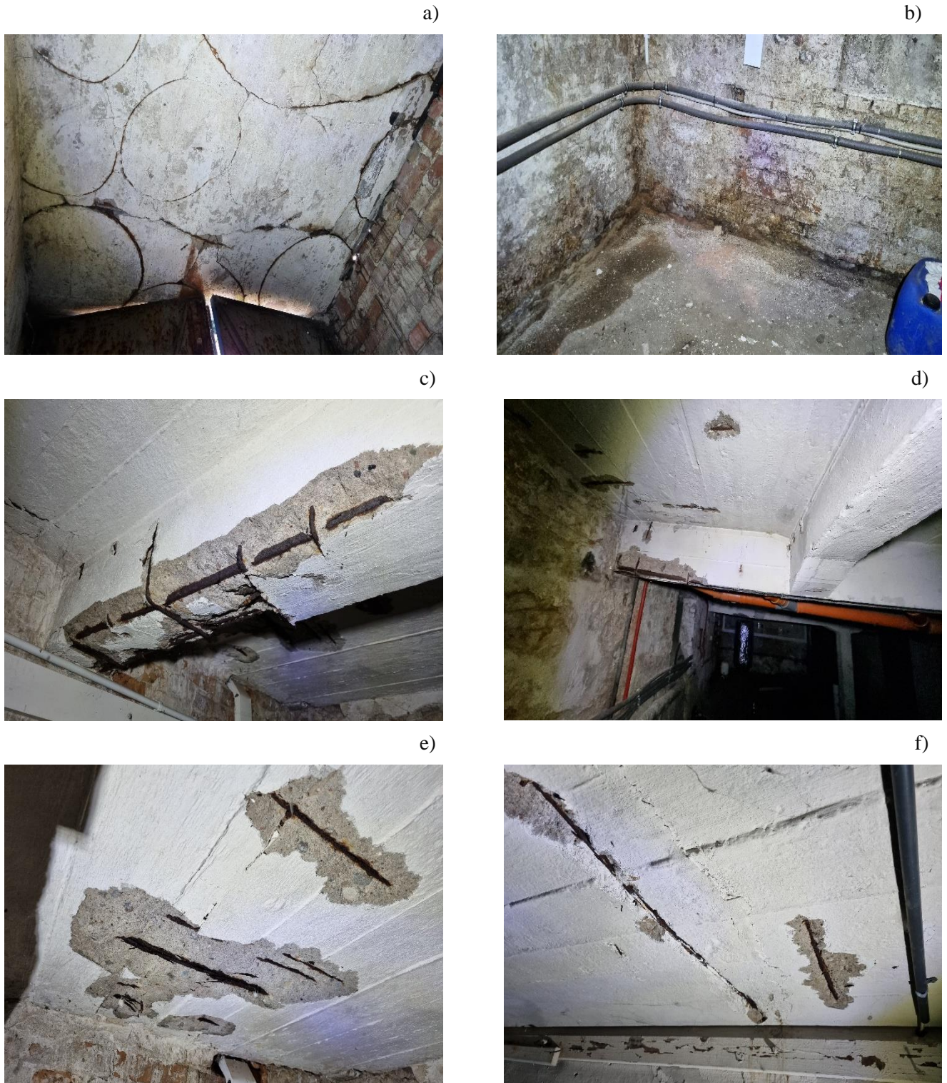
Photo 3. Warehouse Building - elevations: a), b) south-eastern, c), d) south-west Warehouse Building - basement: a) view from the bottom of the ceiling above the annex, b) dampness of the external walls, damage to the concrete cover of the reinforcing bars: c) , d) beams, e), f) ceiling slab
