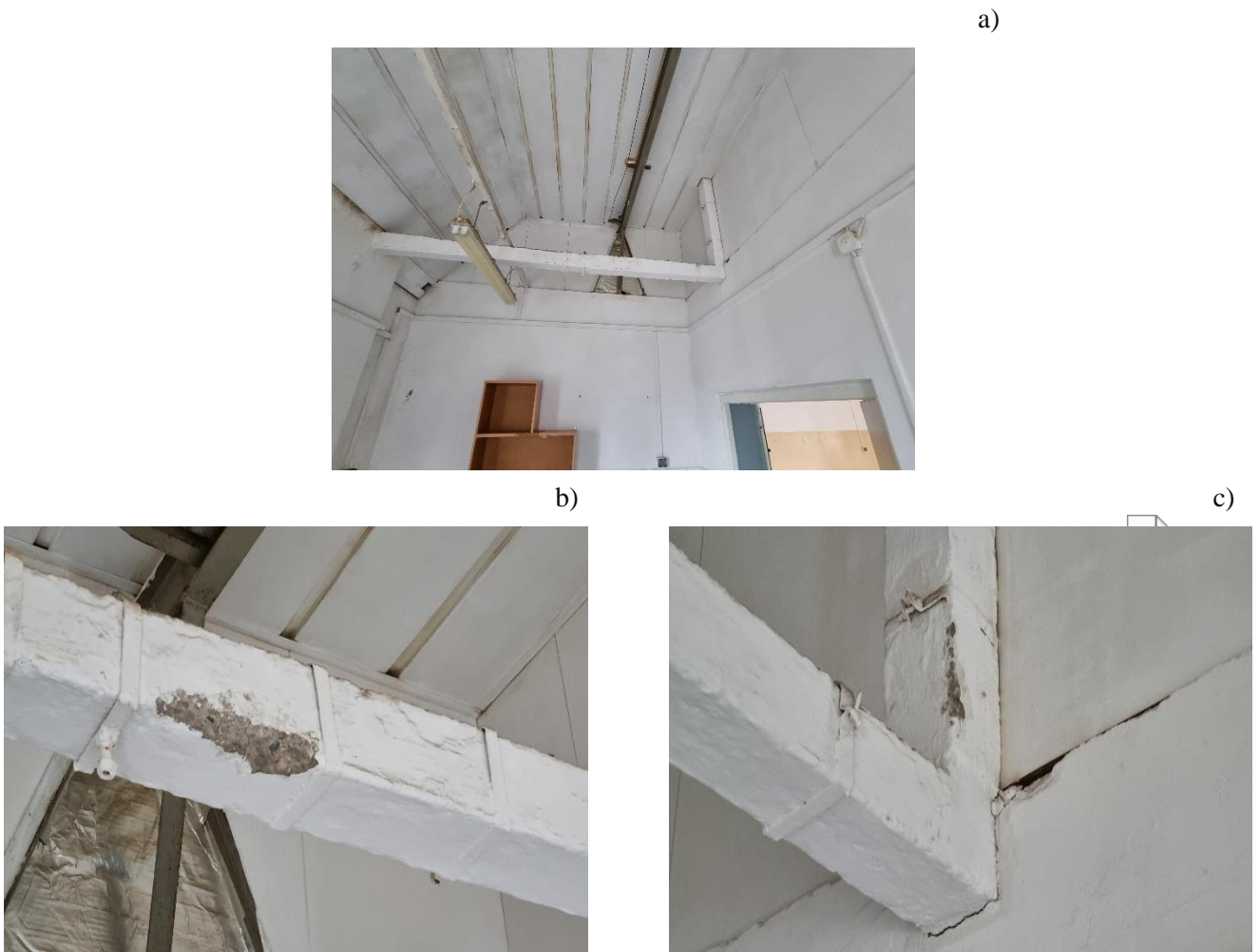
Photo 5. Warehouse building - reinforced concrete tie in the view from the rooms on the ground floor: a) general view, close-up: b) horizontal element - horizontal tie, c) vertical element - post
