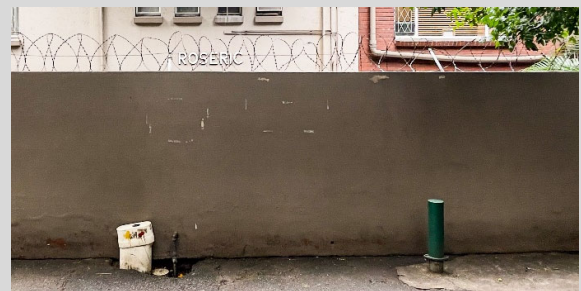
Figure 5-23- Roseric (67 Lena Ahrens Rd.) The rather uncoordinated and considered addition of servicing elements. To the left is a water meter in a ‘tamper proof’ housing that has evidently been tampered with. To the right is a stub column for telephonic infrastructure. As can be seen by the pavement repairs, these are treated in an ad-hoc manner.
