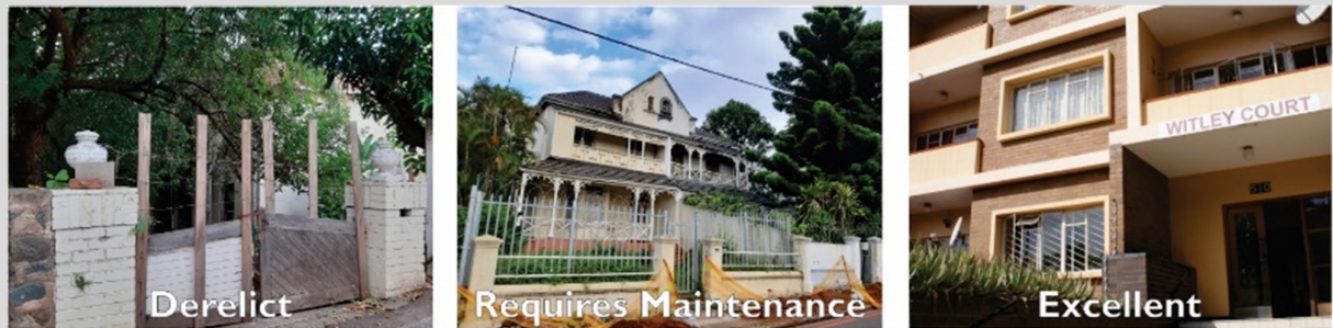
Figure 5-10 -: A selection of buildings of different conditions of their current fabric found in the overall study area. From left to right: 79 J.B. Marks Road (derelict), 76 & 78 Hunt Road (requires maintenance), and Witley Court (510 Che Guevara Road – Excellent).
