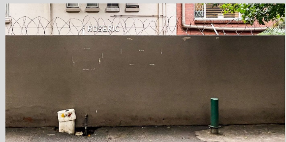
Figure 5-23- Roseric (67 Lena Ahrens Rd.) The rather uncoordinated and considered addition of servicing elements. To the left is a water meter in a ‘tamper proof’ housing that has evidently been tampered with. To the right is a stub column for telephonic infrastructure. As can be seen by the pavement repairs, these are treated in an ad-hoc manner.
