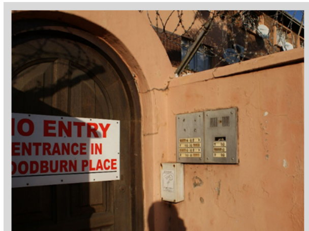
Figure 2-57 - Hennet Court, 1955, 328 Che Guevara Rd. The lack of maintenance, subsequent installation of visually intimidating security measures such as the barbed wire that is rusting, and the reduction of street surveillance through the construction of a solid boundary wall leads to a compromised image of a sense of security on the street.
