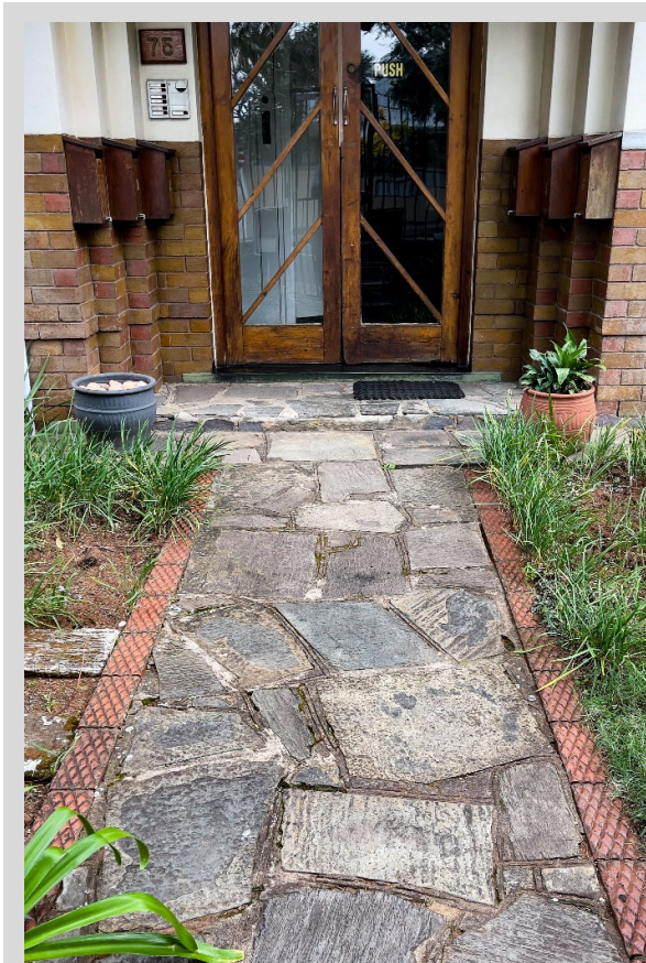
Figure 5-35 - Wilfton (75 Ferguson Rd.) The slasto garden path with clay brick border echoes the use of 'natural materials' along with the face brick plinth and timber framed entrance doors.
