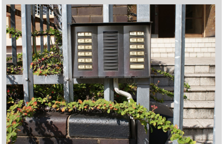
Figure 2-58 - Targeting hardening include physical barriers, such as this palisade fence and also landscaping, such as this thorny groundcover. The advantage of using soft landscaping in a target hardening fashion is that it does not appear to be a security device, but adds to the overall attractiveness of the streetscape.
