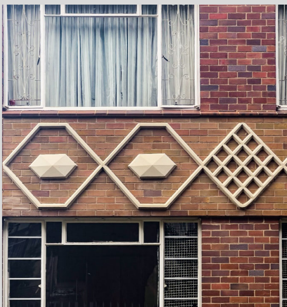
Figure 5-65 - Retford Hall (151 Lena Ahrens Road). A composition in varying face brick panels. The individual original windows with steel frames show a variety of burglar bars, which detracts from the consistency of the visuals. The windows are in a slightly recessed panel with a continuous quarry tile cill that runs along the entire panel, including the brickwork portion between windows. The applied decorations standing proud of the façade is fairly rare in the study area.
