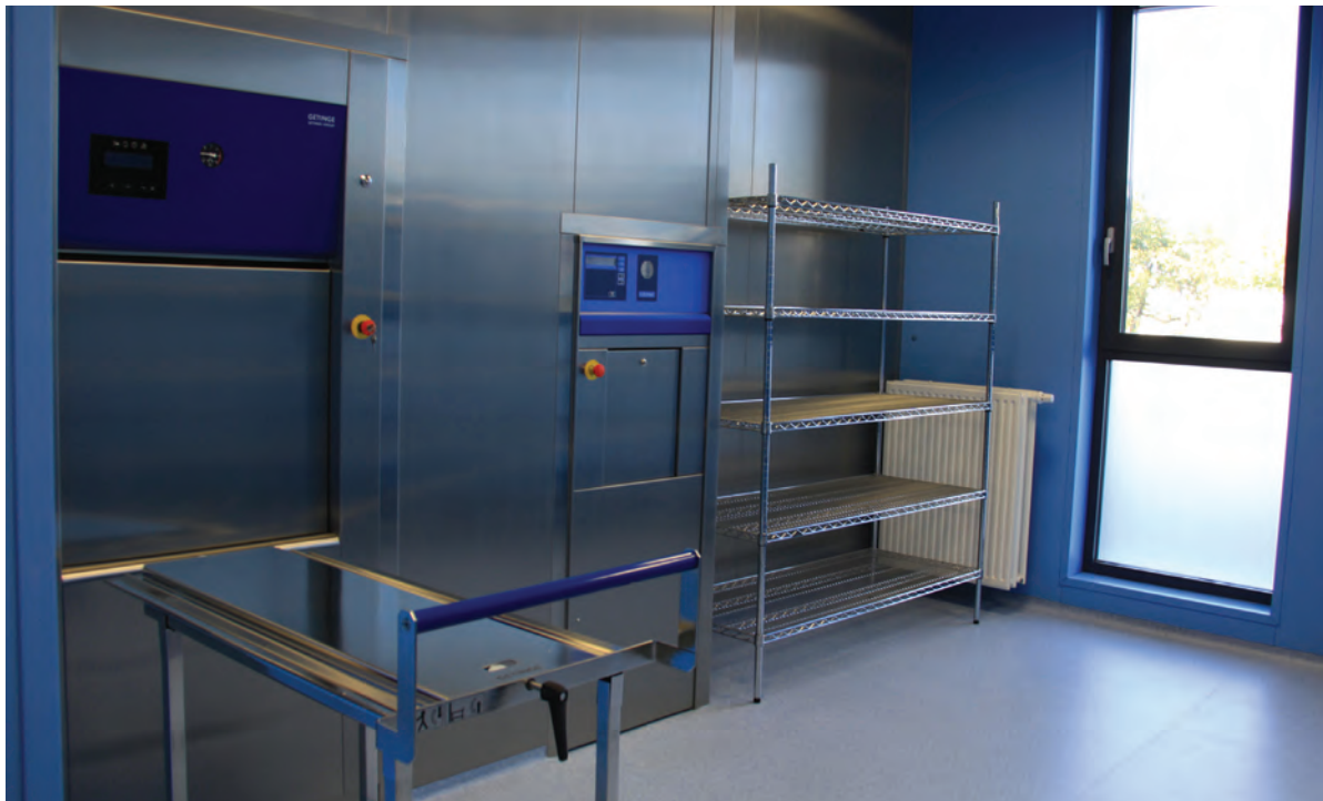
Photograph 6.4.3 A central sterilisation unit (physical separation of the dirty, clean and sterile sections allows for reducing the possibilities of secondary contamination of medical instruments); photographed by the Author 2016
