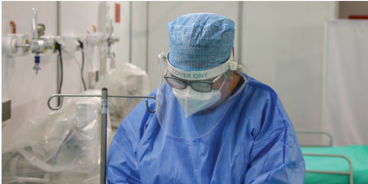
Photograph 2.3.1 An example of air disinfection with the use of UVC lamps used in order to maintain the assumed hermeticity of the rooms; a temporary hospital at AMBEREXPO in Gdańsk; designed and photographed by the Author, 2022
