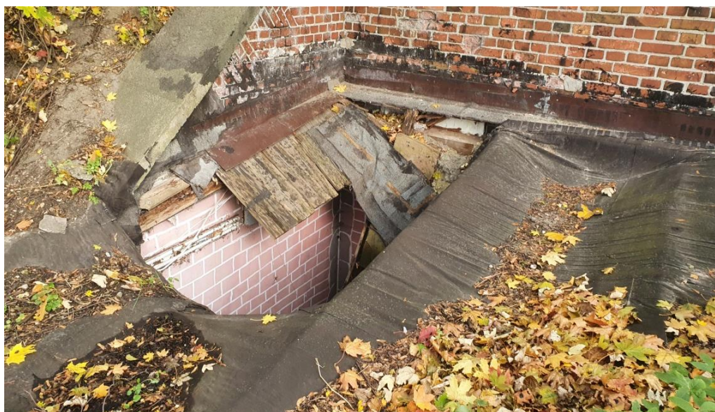
Fig. 15. Moisture damage to ceramic masonry as a result of water flooding caused by the collapse of a moisture-damaged and biologically corroded wood-framed roof: a) view, b) close-up (photo: Maciej Niedostatkiewicz)
