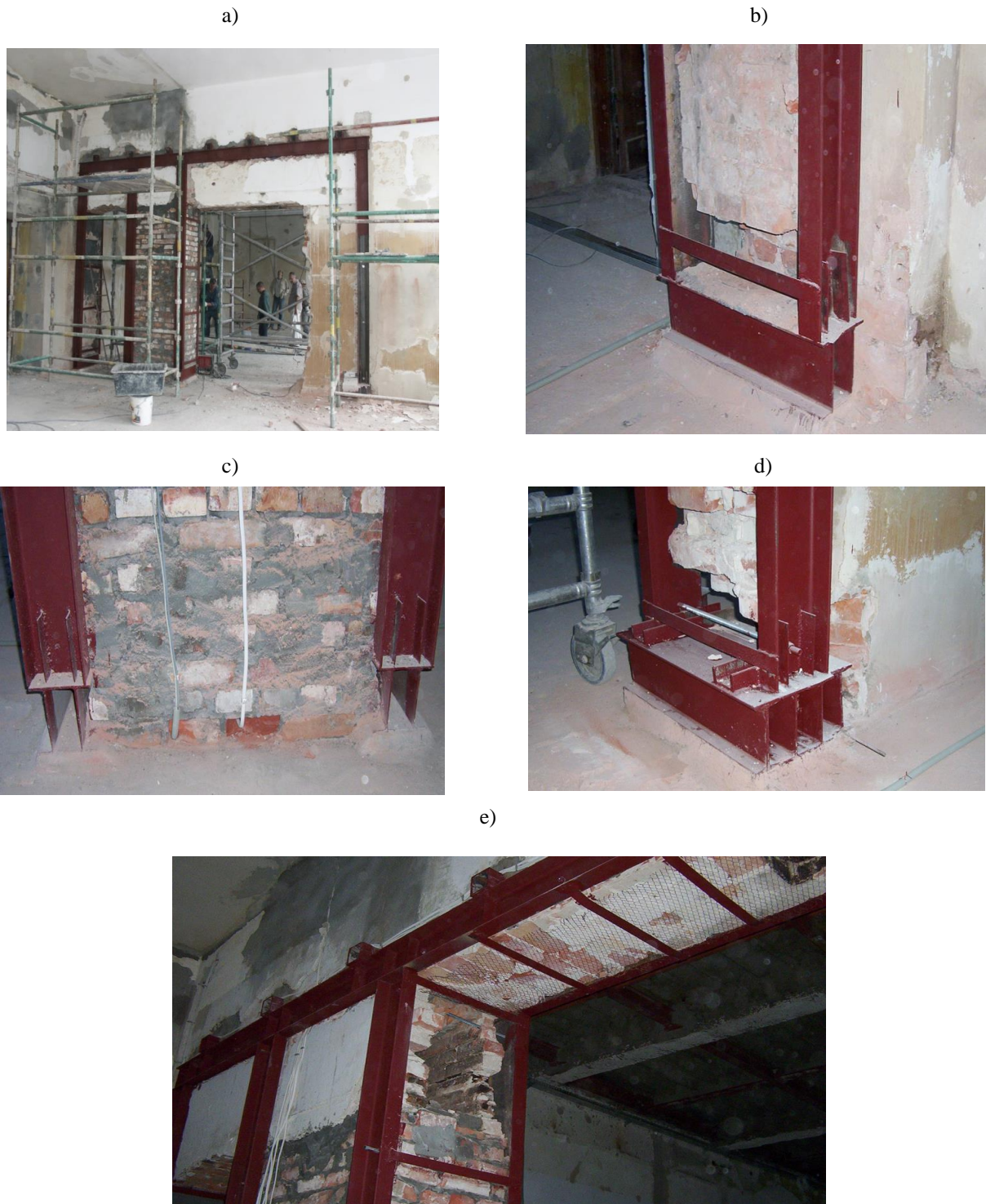
Fig. 17. Making door openings in the inner wall of solid ceramic brick: a) view of the steel frame, b), c), d), e) construction details (photo: Tomasz Majewski)
