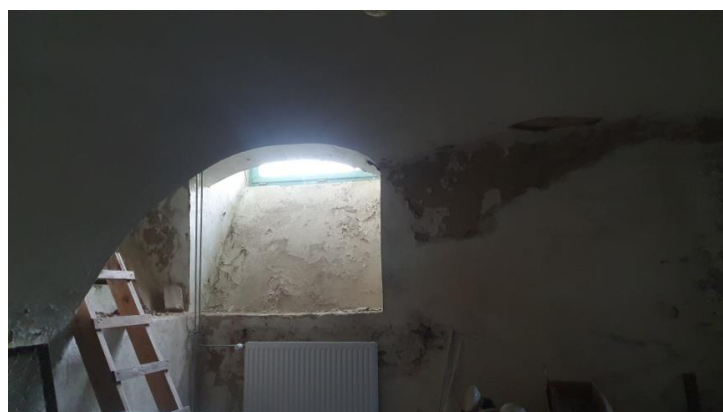
Fig. 7. Dampness of the external wall made of solid ceramic brick caused by the lack of vertical damp proofing in the part sunk in the ground (photo: Maciej Niedostatkiwicz)
