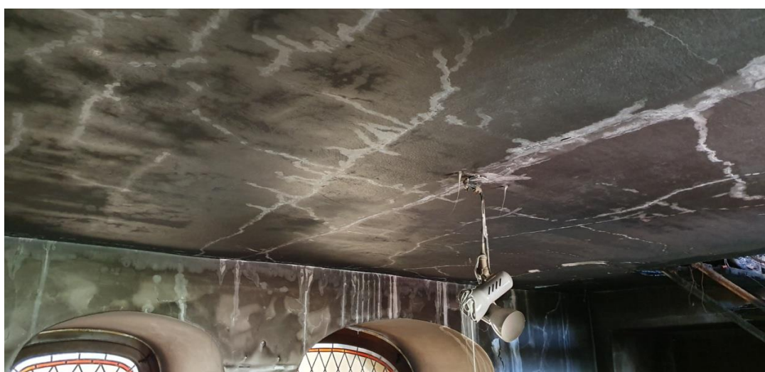
Fig. 5. Fire damage to solid ceramic brick wall and ceiling on wooden beams, visible cracks in plaster on wall and ceiling (photo: Maciej Niedostatkiewicz)
