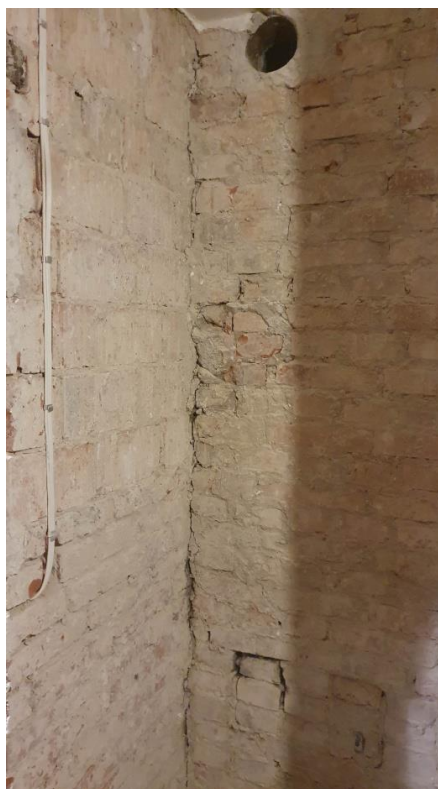
Fig. 13. No masonry bond between transverse and longitudinal interior walls made of ceramic solid brick (photo: Maciej Niedostatkiwicz)
