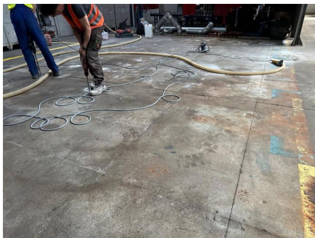
Fig. 3. Degraded concrete industrial floor (Example 1) during repair: damage inventory, removal of mounting anchors [38]
