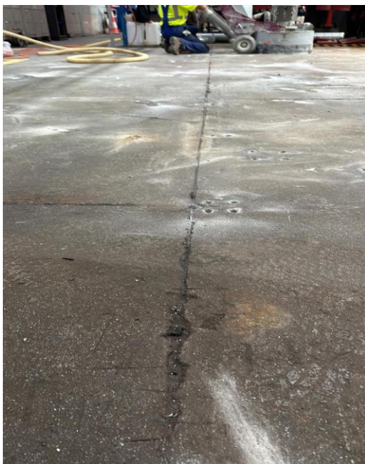
Fig. 2. Degraded concrete industrial floor (Example 1): visible wear of the top layer, mounting anchors left over from equipment removal, and shrinkage joint damage [38]
