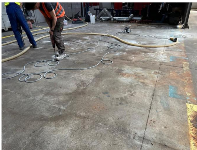
Fig. 3. Degraded concrete industrial floor (Example 1) during repair: damage inventory, removal of mounting anchors [38]
