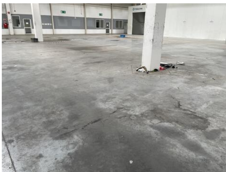
Fig. 14. Concrete industrial floor (Example 4) before renovation: damaged upper floor surface due to improper use of cleaning agents [38]
