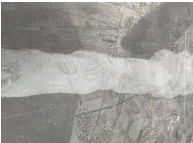
Fig. 6. Concrete industrial floor (Example 1) during repair: making an addition to the basin formed after the removal of the process channel [38]
