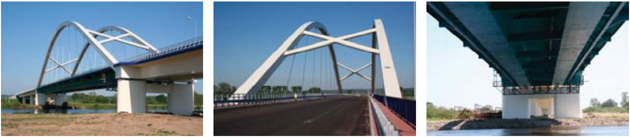
Fig. 7. Construction of the arch stayed span of the bridge in Gorzów Wielkopolski
