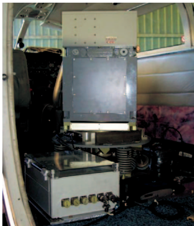
Fig. 1. The GT-1A gravimeter installed on Cessna 404 plane [12]
