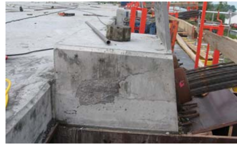
Fig. 3. Damaged cantilever no. 4 after prestressing
