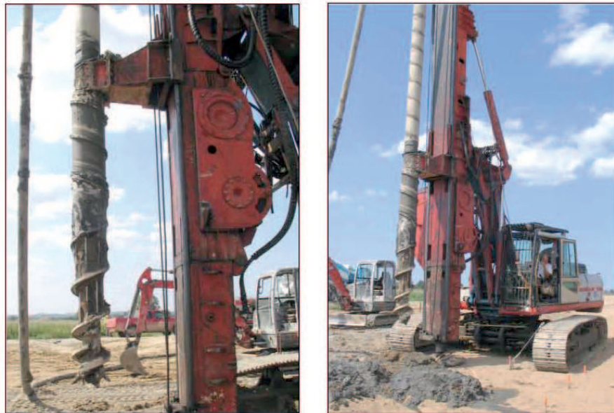
Fig. 3. Screwing auger and piling machine used in the experiment. Rys. 3. Świder i palownica do wykonywania badanych pali i kolumn
