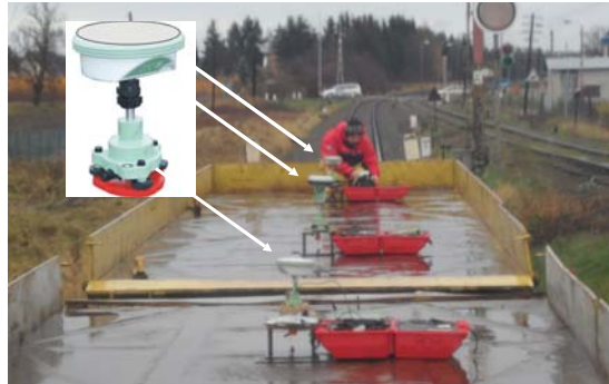
Fig. 3. GPS Total station receivers location on the platform [own photo]
