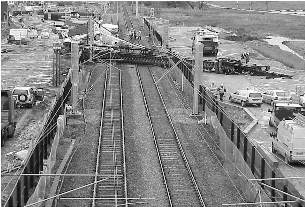
Rys. 8. Awaria na placu budowy Channel Tunnel Rail [4]
