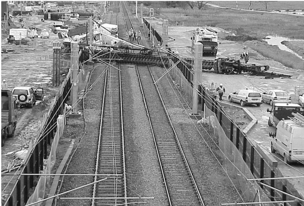
Rys. 8. Awaria na placu budowy Channel Tunnel Rail [4]
