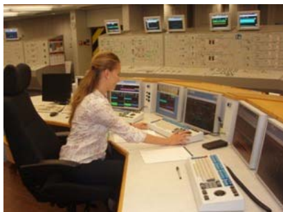
Fig. 5. Simulator of control room
