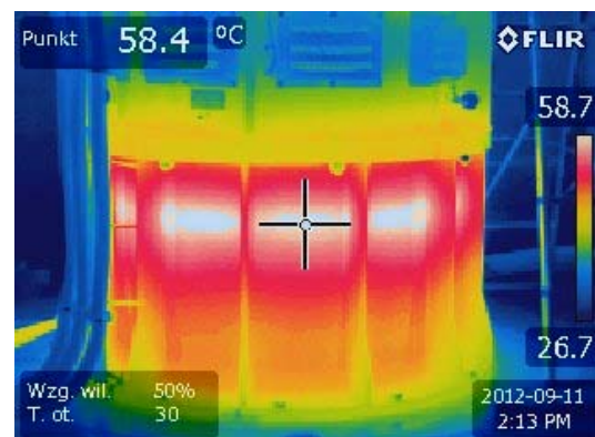
Fig. 6. The temperature distribution on the external surface of the gear housing.
