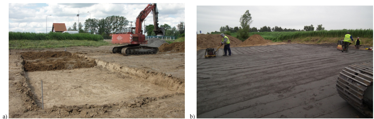
Fig. 4. Construction stages: (a) preparation – removal of soft soil (b) compaction of single layer of dike body
