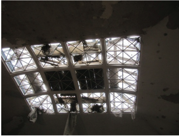
Fig. 4. Reinforced concrete grid of the skylight as seen from the inside of the Seaport Hall
