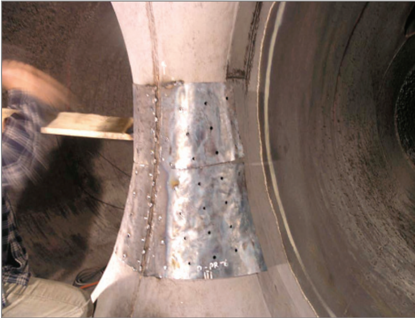
Fig. 16. Quadrangular components of the reinforcement in the process of tacking along centerline of the branch.
