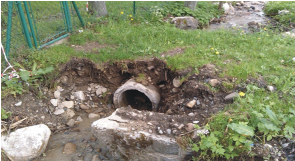
Fig. 1. Scour caused by storm water at aculvert inlet (Kuźnice, Poland, May 28, 2014)
