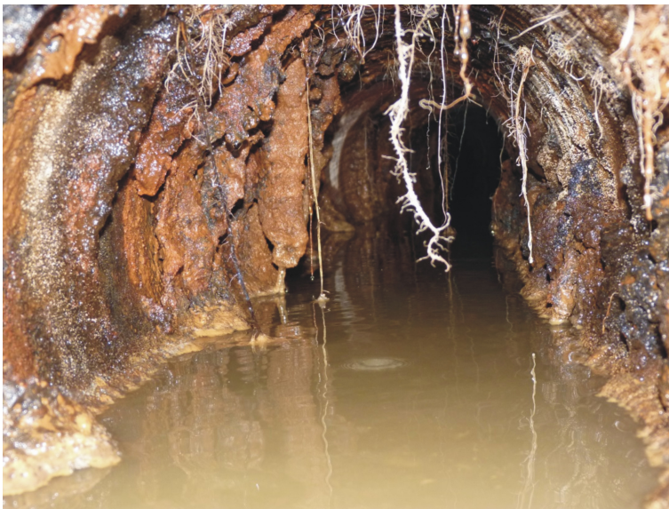
Fig. 4. Ferruginous substance in a pipe
