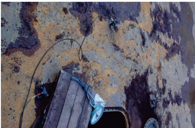
Fig. 12. View of the deck in the vicinity of the tank No. 11 of the Naval Shipyard Co floating dock
