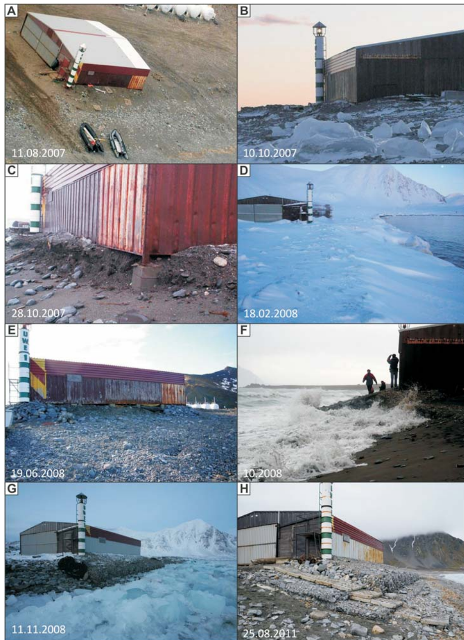
Fig. 8. The effects of coastal erosion processes in the area of harbour building of Polish Polar Station – “Banachówka” and methods of its protection. Photo: M. Błaszczuk archive (A–D, F), J. Kwaczyński (E, G), P. Zagórski (H).
