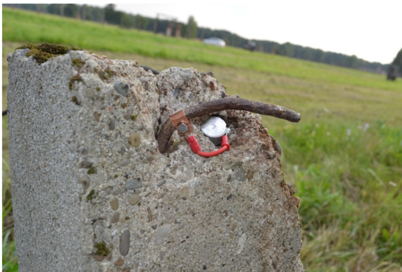
Fig. 7. Pillars located in the former Auschwitz camp protected with sacrificial anodes before applying a new repair mortar: variants with protector buried in soil (a), variant with protector placed directly on reinforcement (b).
