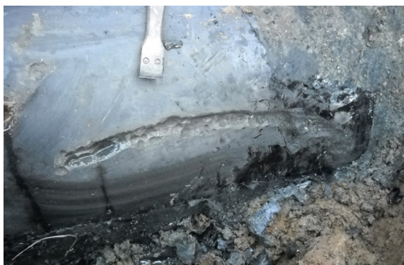
Fig. 2. Zoom on the defect site.
