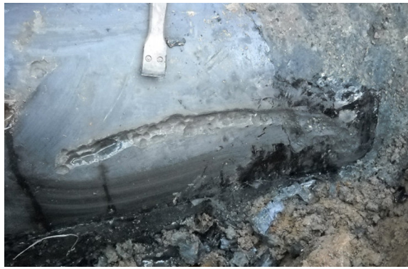
Fig. 2. Zoom on the defect site.
