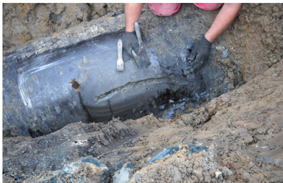
Fig. 1. View of pipeline corrosion failure.
