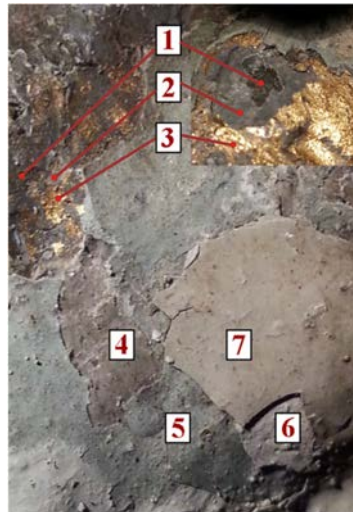
Fig. 7. The surface of decorative metal element of railing bar. The layers of painting coats are numbered consecutively.
