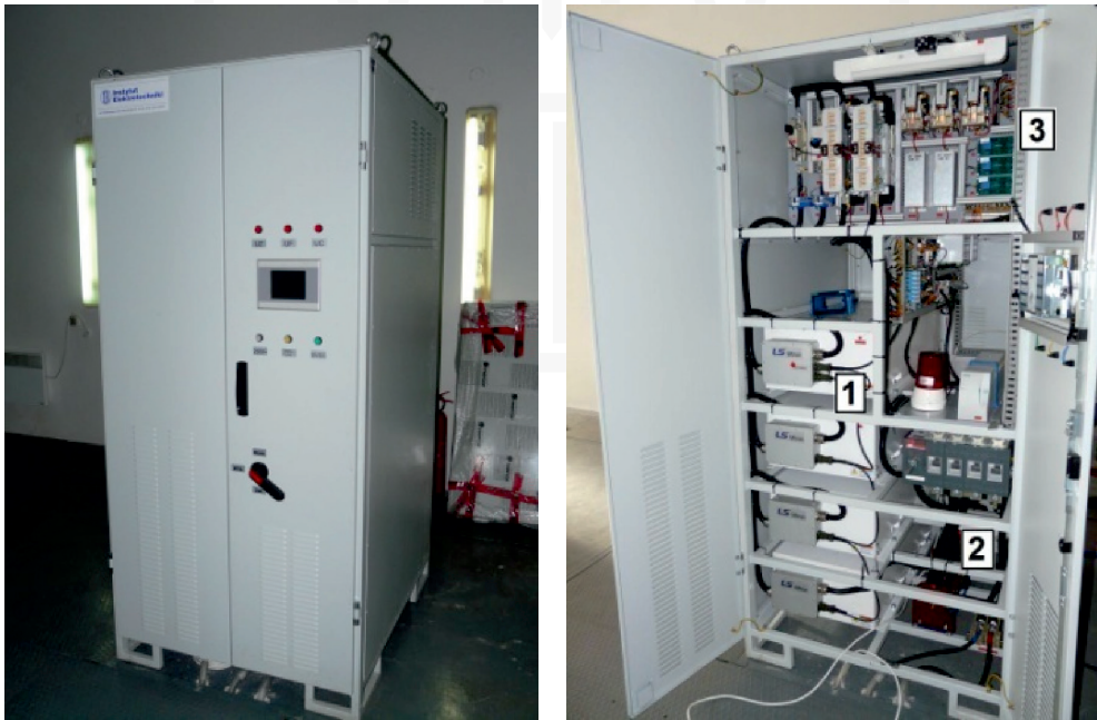
Fig. 5. Supercapacitor energy bank installed in the traction substation Północna in Gdynia; 1 – supercapacitor modules, 2 – DC/DC converter with the controller, 3 – protection modules and filter
