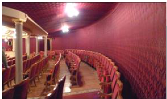
Fig. 8. The underbalcony space in the Lviv Opera House hall prior to installing the sound diffusing structures. The walls and ceiling were covered with a textile tapestry.
