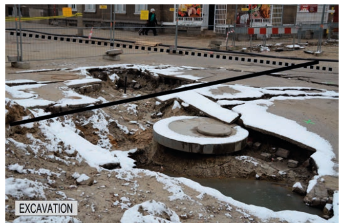
Figure 13. Close-up of the Gdańsk 2013 pipe failure area Dotted lines indicate road edges while solid line indicates the axis of the pipeline
