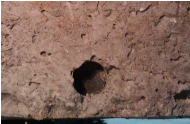
Fig. 9. Detail of slab C-2 after its failure
