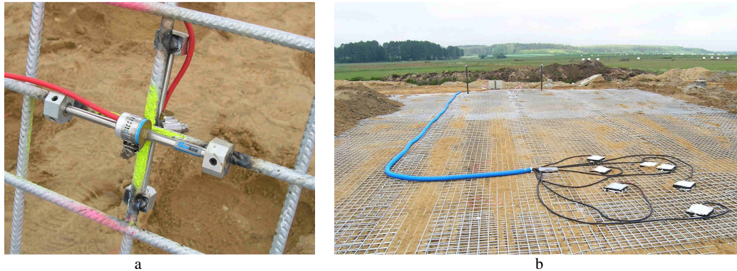
Fig. 6. a. Strain gages on the steel grid; b. Location of the protected sensors before backfilling
