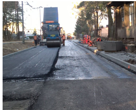
Figure 4. Poor quality and lack of tack coat on the asphalt base course. Road R3L.
