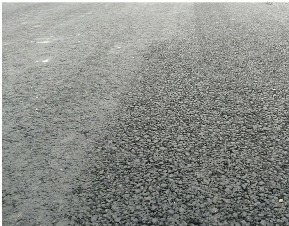
Figure 3. Surface of the lower asphalt base course AC22P. Non-homogenous surface. Road R1S.
