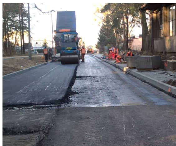
Figure 4. Poor quality and lack of tack coat on the asphalt base course. Road R3L.
